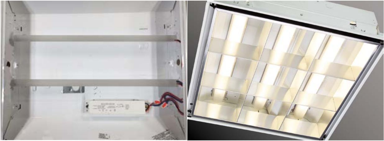
LED Strips and driver installed in 2 x 2 Troffer Completed Retrofit with ballast cover and Trim Reinstalled
